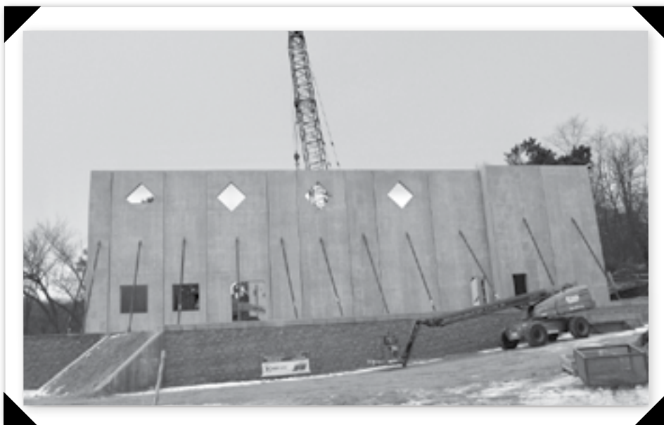
Decorative and insulated wall sections manufactured locally by Huffcutt Concrete, Inc. were lifted into place by a crane beginning January 19.
